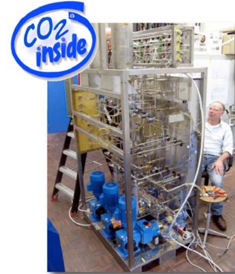
CO 2 cooling system
